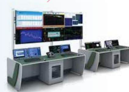
Central Control Room
